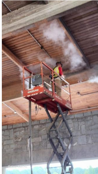
Concourse/ Platform- Ceiling Dry Ice
